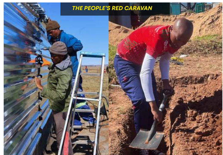
FREE STATE GLADSTONE COOP CONSTRUCTION
